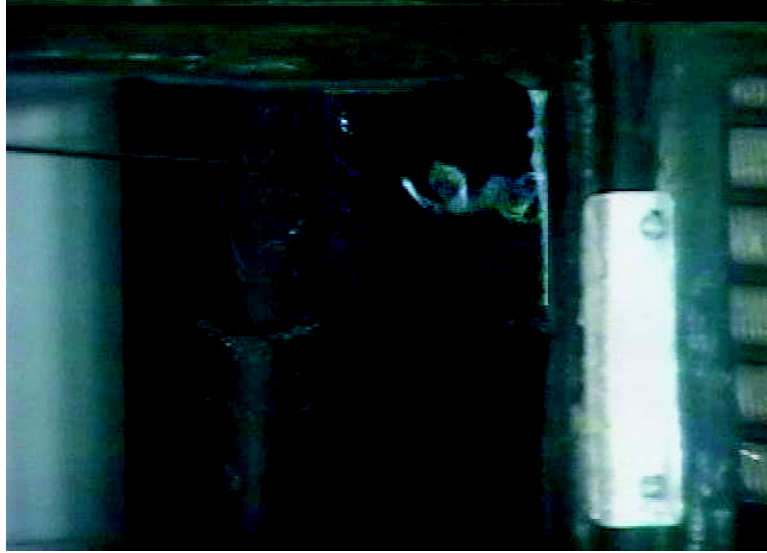
Figure 4.2: Jet flow pattern at the exit of a fan upstream of evaporator
